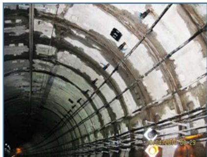
纵缝和环缝渗漏
