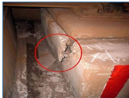
轨下支撑块破损
